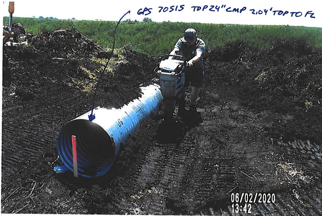
PICTURE # 3640 IS LOOKING SOUTH SHOWING BACK FILL SOIL AROUND 24" CMP WITH CREW USING JUMPING JACK COMPACTOR TO COMPACT SOIL AROUND CMP.
