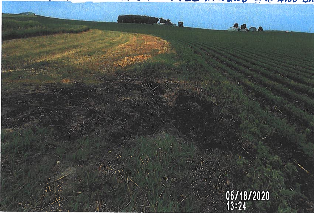
PICTURE # 3839 IS LOOKING NW SHOWING AREA ALONG FIELD NW OF NEW 24" CMP WHERE GOOD SOIL WAS EXCAVATED FOR BACK FILL AROUND CMP AND BACK FILLED
