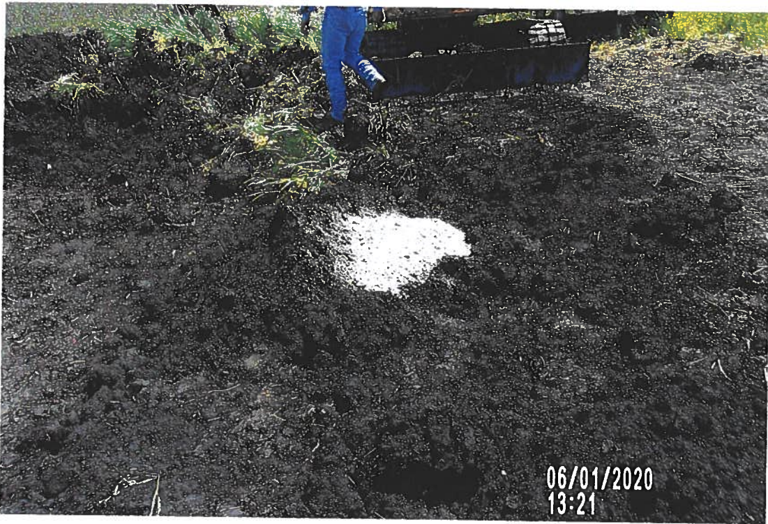
PICTURE #3621 IS LOOKING NE SHOWING 2 BAGS OF 60 LB QUIKRETE CONCRETE & 2.0'x2.0' PIECE OF FABRIC PLACE OVER EXISTING HOLE TORE IN TOP OF EXISTING 24" CMP.
